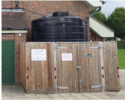
Rainwater Harvesting Tank
